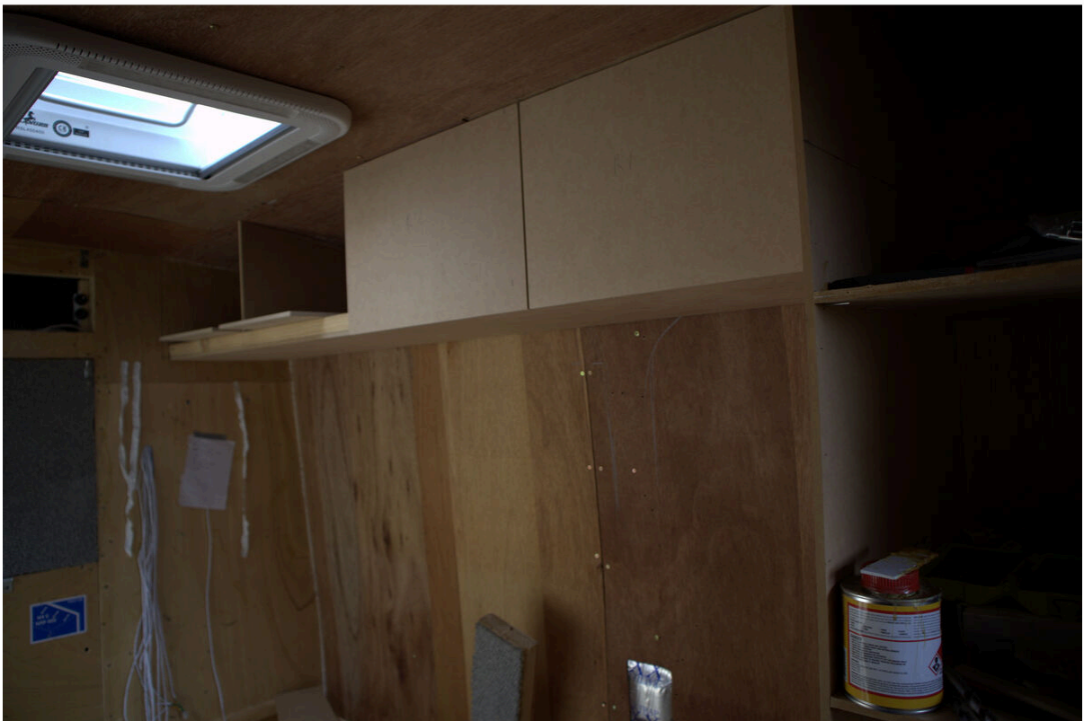
Seating area cupboards being fitted with framing cut in half to save weight
