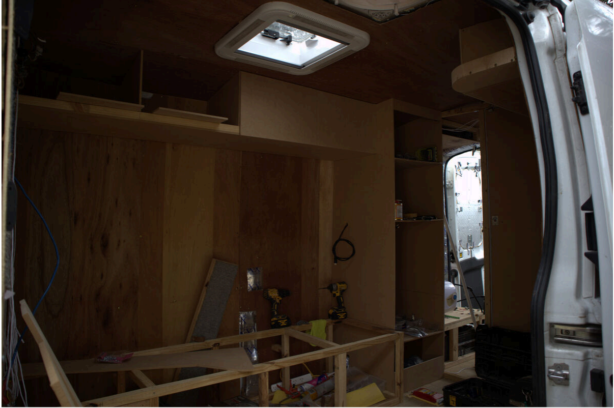
Main cupboard unit going in — built outside the van then slotted into place
